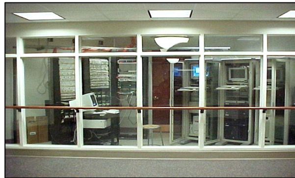
IT Server Room
